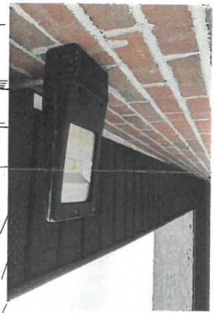
▲ New LED Wall Mount (6 fixtures total)
