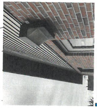
■ Old Wall Mount Lights (2 fixtures total)
